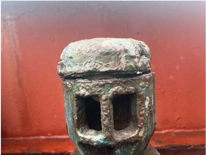
Corrosion of air pipe head
