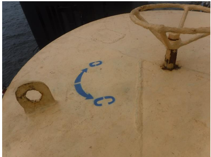
Incorrect marking of ventilation open/close direction
